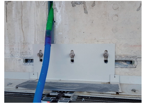
Figure 23: Use of post-installed anchors due to wrong positioning of the anchor channel
