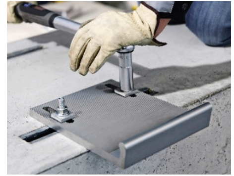
Wrong installation torque
